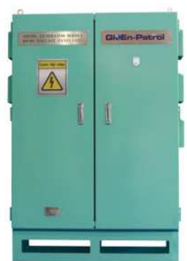
UV POWER SUPPLY PANEL
