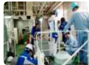
Pump piping line check
